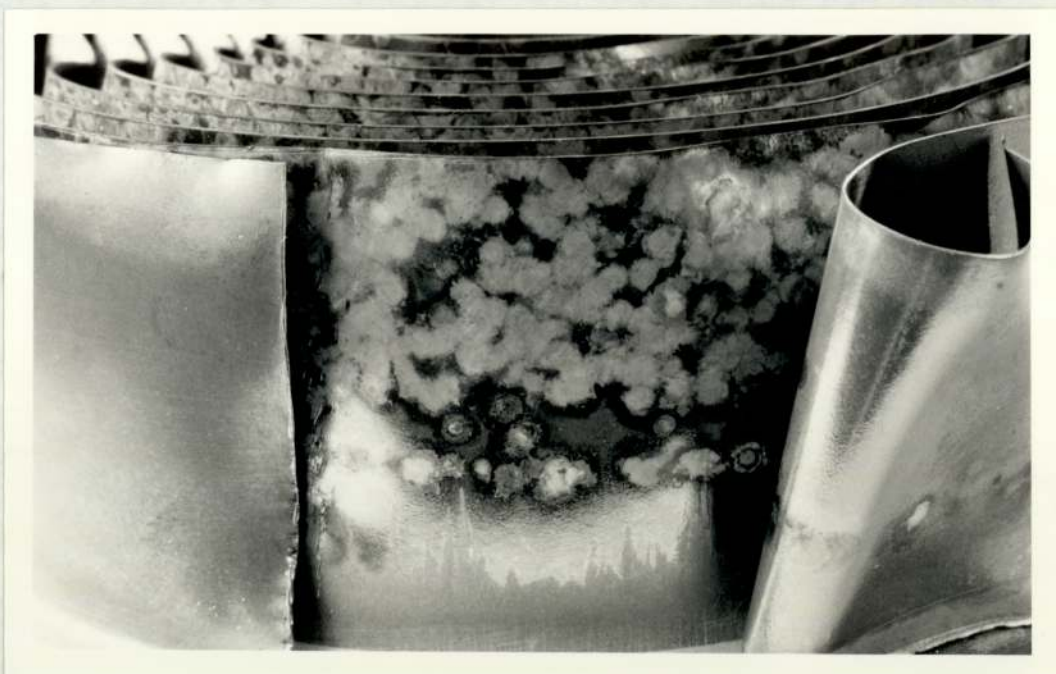
Fig.6.2 Surface Damage Produced By Commercial 'Spot-Knocking' Of HV Capacitor (failed in service)
