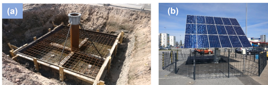
Fig. 9. PV system with solar tracker - (a) system foundation (b) complete operational system.
