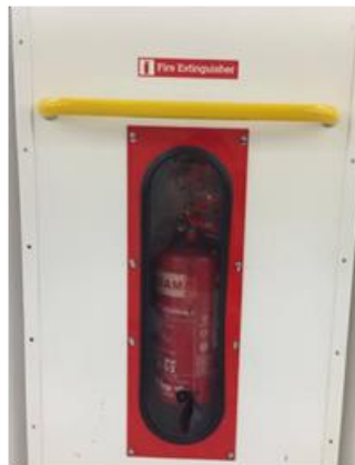
Figure 6: Fire extinguisher casing on-board metro
