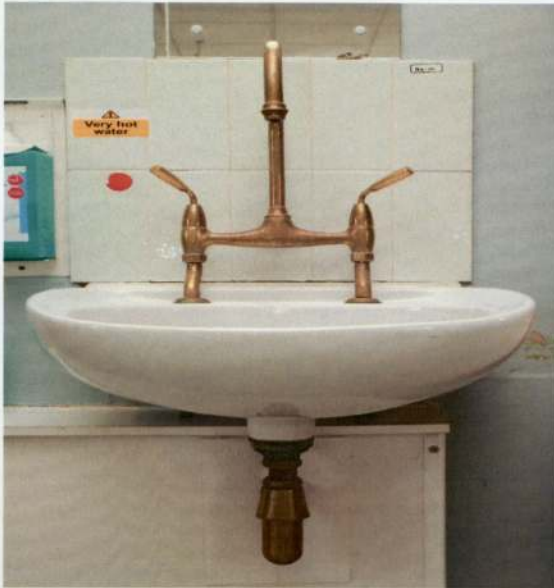
Copper sink waste fittings
