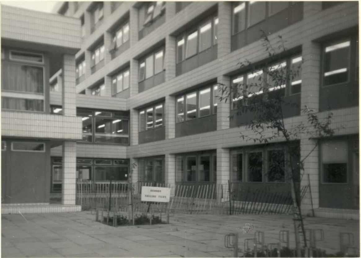
Plate No. 5.14 Elevation - showing unsatisfactory white tile finish
