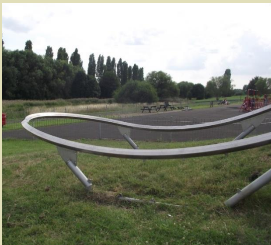
Figure 7: Broken play equipment at Babbs Mill
