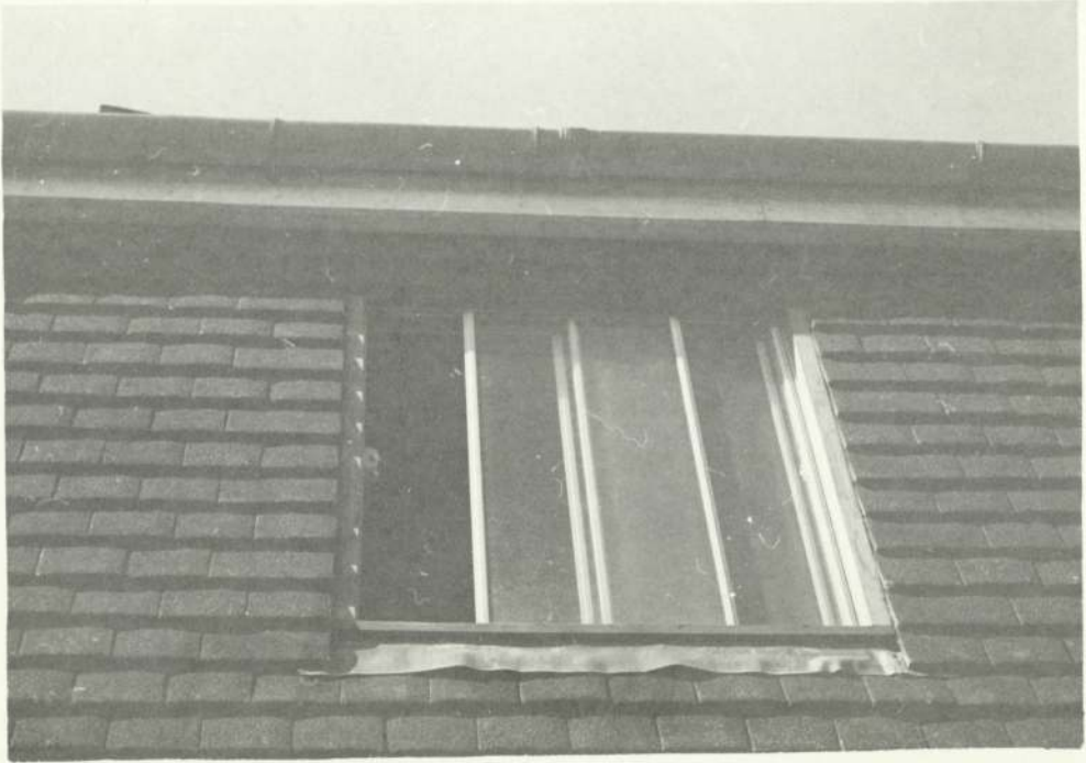
Details of eaves and window inserts using two part fascia and soffit
