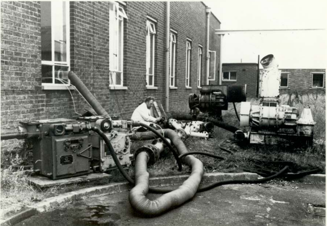
FIG 29 AIR SUPPLY SHOWING POSITIVE DISPLACEMENT BLOWERS AND ELECTRICAL CONTROL UNITS
