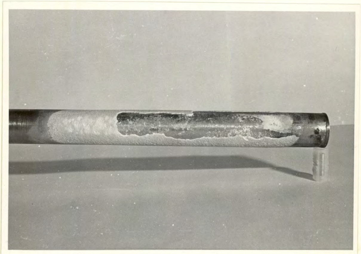
TUBE WITH SCALE PARTIALLY REMOVED SHOWING RELATIVE THICKNESS OF DEPOSITS AND AREAS OF ADHESION TO TUBE
