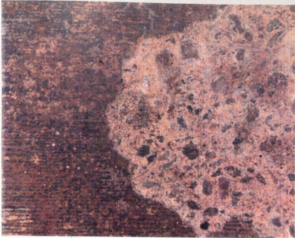
Plate 4.5 - Cracking and Scaling of Poned Surface (Potassium Acetate) x 1 Mag.
