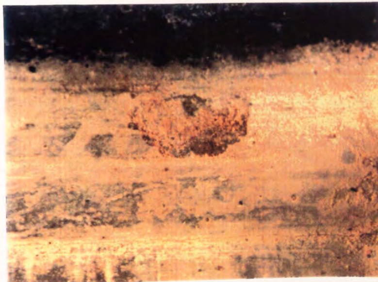
Plate 4.13 - Damage on Side Wall of Ponded Slab Reservoir (Commercial grade CMA) x 1.5 Mag.
