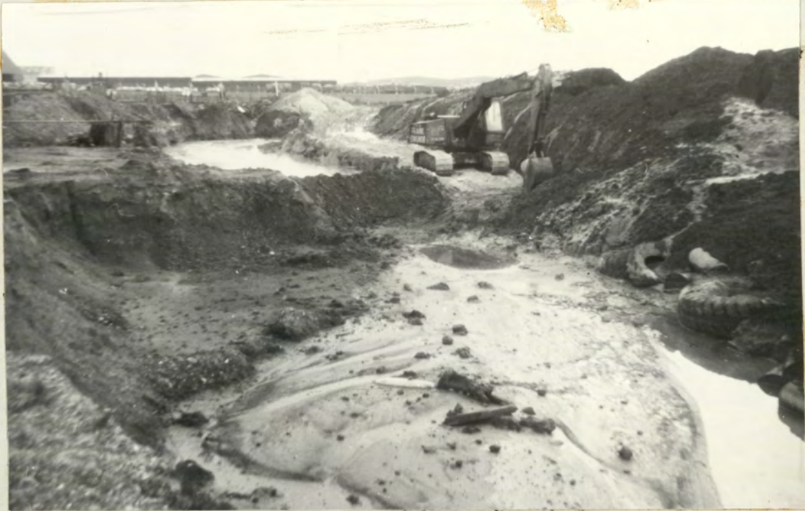
FIGURE 3.7. Large Scale pH Adjustment Process, Mechanical grab feeding sludge into acid lagoon in a pretreatment process.
