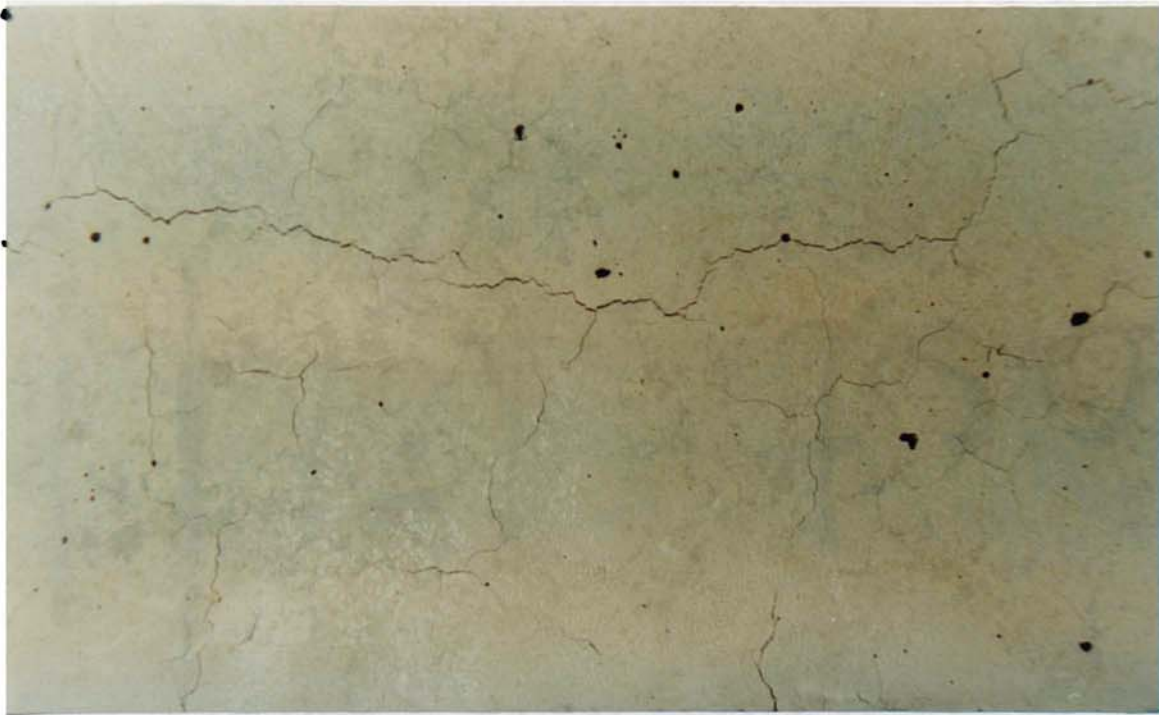
Figure 8.4 Photographs to show cracking along a test beam
