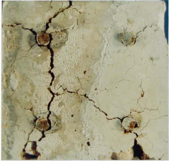
Figure 8.3 Photographs to show severe cracking at the ends of test beams
