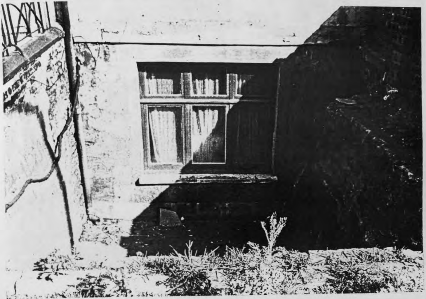
FRONT AREA OF 56 BARNSBURY ROAD INCREASED IN fig. 5.19 SIZE BY THE DEMOLITION OF THE VAULTS
