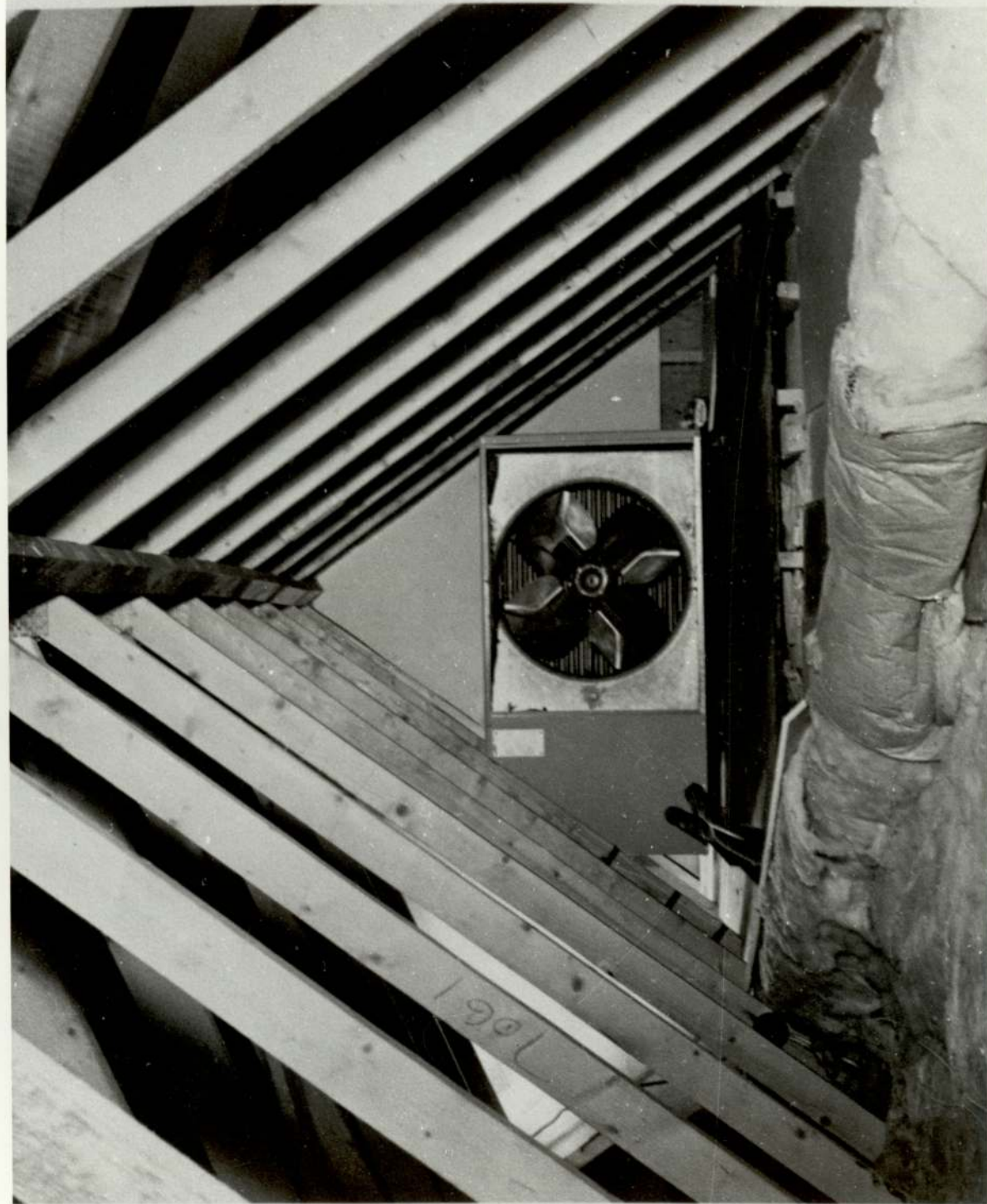
Photograph 2.3: The heat pump in the roof space, its safety grille removed.
