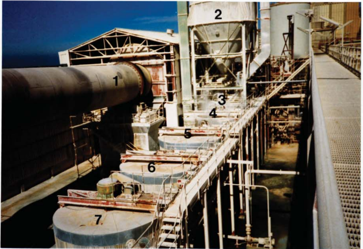
Figure 7.3: General arrangement of the equipment in the chemical recovery zone. (Courtesy of SOPORCEL — Leirosa, Portugal)
