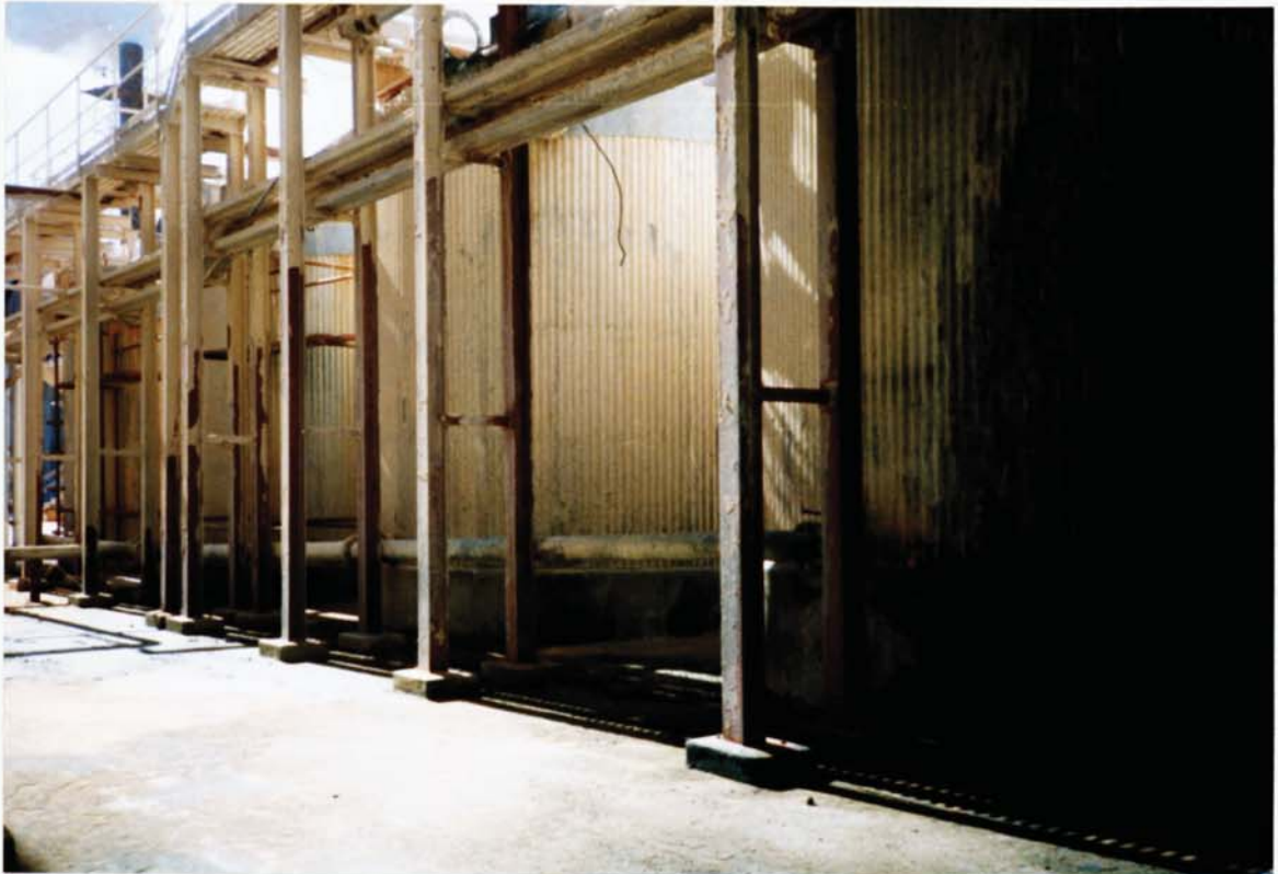
Figure 7.4: Side view of the causticizing tanks. (Courtesy of SOPORCEL — Leirosa, Portugal)
