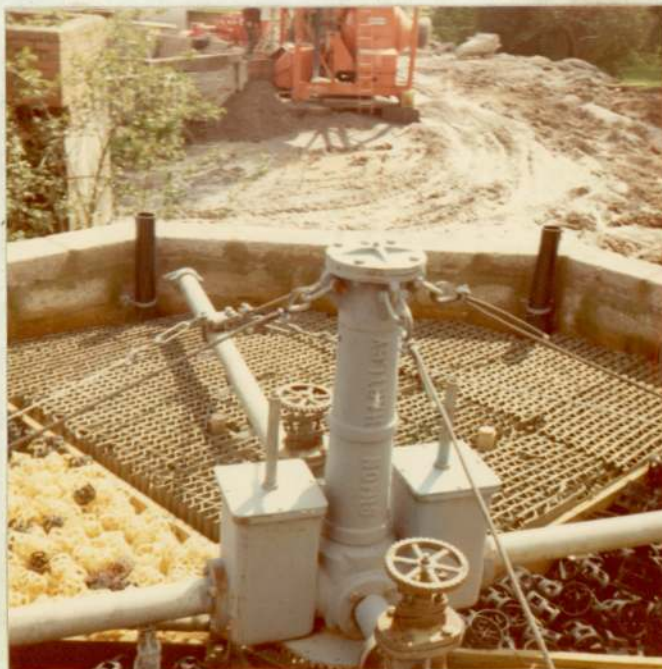
Distribution System to Filters.
