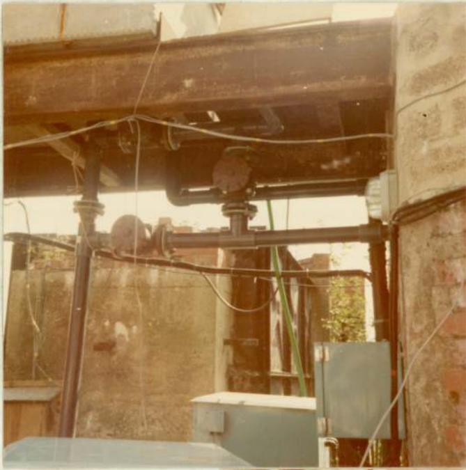
Plate 4.6 Header Tank Distribution Pipework.
