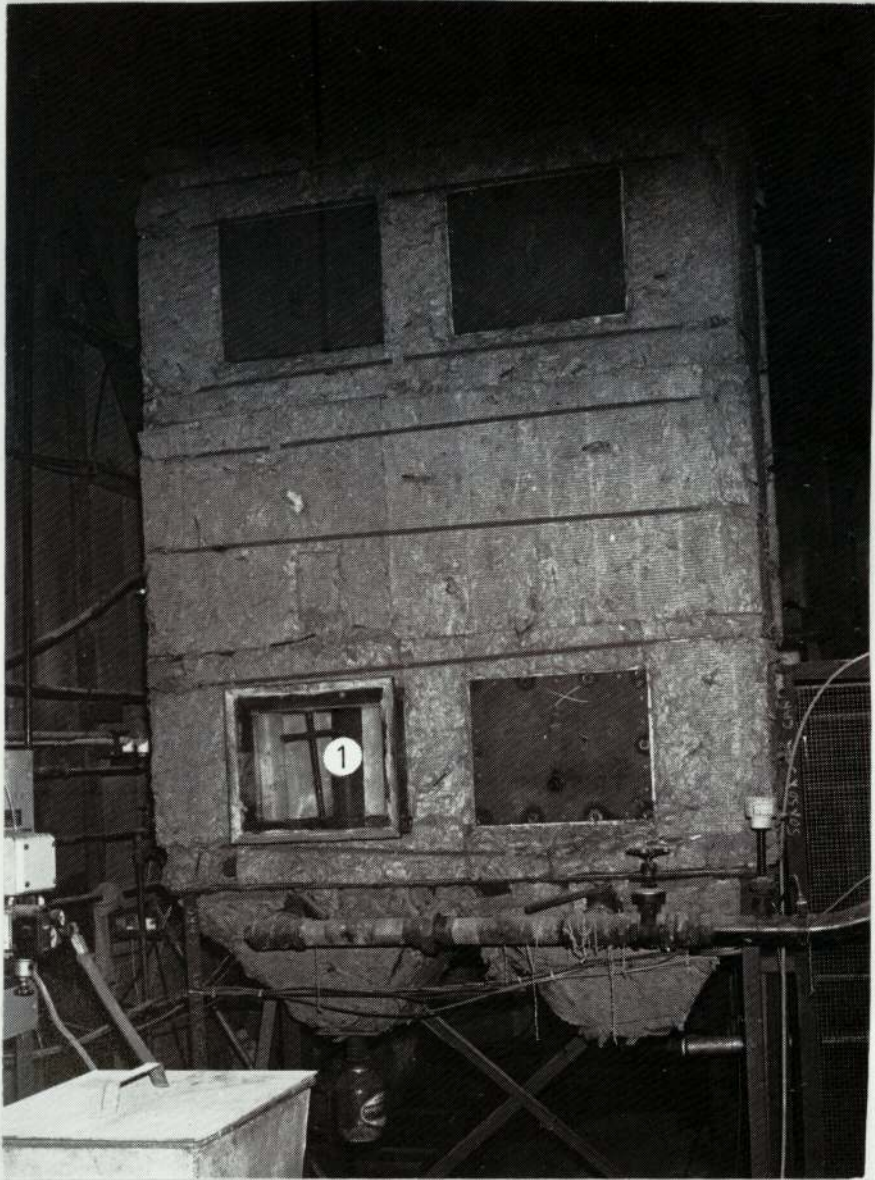
FIGURE 5.9 : The twin-compartment Bag Filter. The reverse air cleaning arrangement is out of view but the pulse air cleaning mechanism can be seen(1) .
