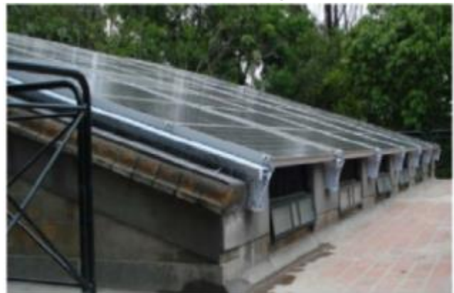
BIPVT fitted on the rooftop
